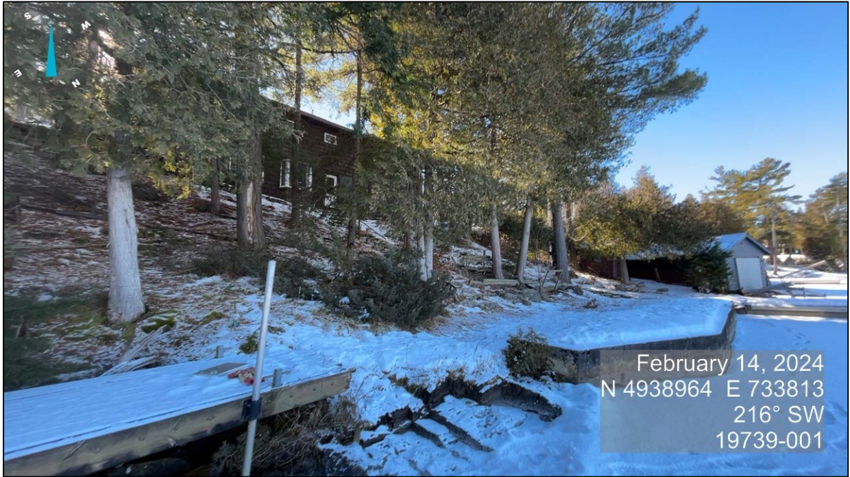
Photo 7 Exposed bedrock between wooden decking and concrete pier at toe of slope.
