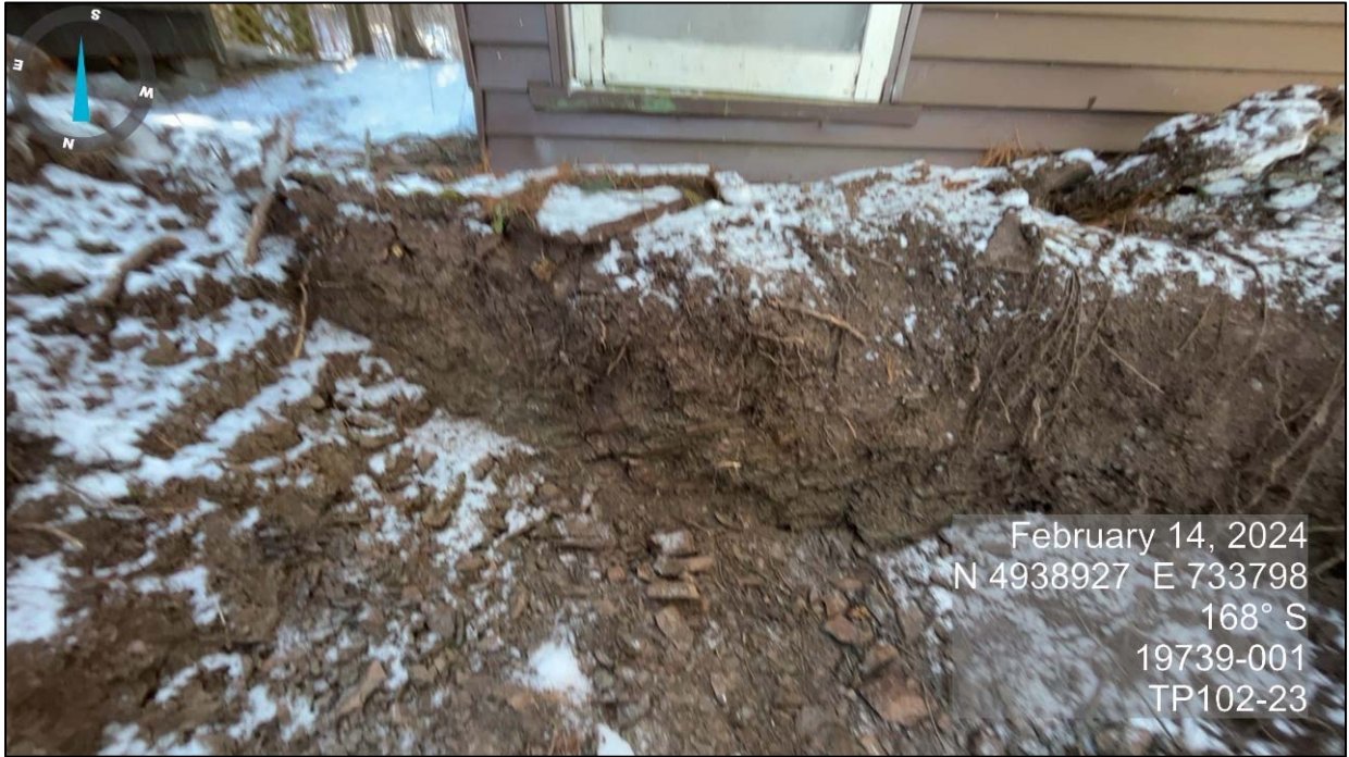
Photo 3 TP102-24. Weathered fissile bedrock overlying competent bedrock. Weathered bedrock has been excavated and removed from test pit.
